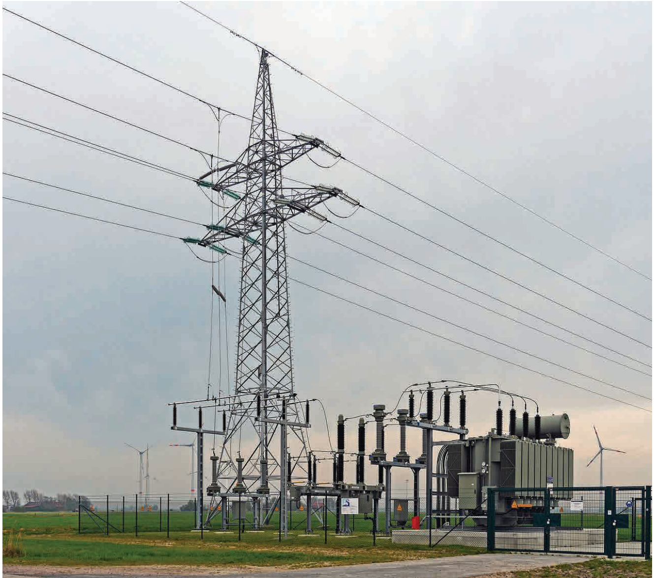
An example of a 72kV vacuum circuit breaker installation, connecting a renewable energy plant with a transmission network.
